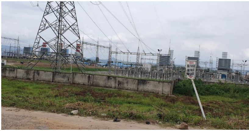
[Abandoned Steel Manufacturing Factory, Nigeria]
